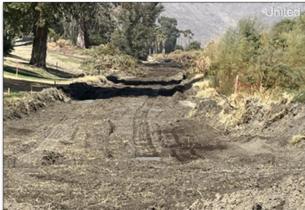
Clearing and grubbing at multiple locations and removing trees that are in conflict with JPCP.
