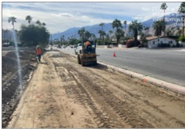
Grading and balancing dirt on the east side of Sunrise Way in Palm Springs
