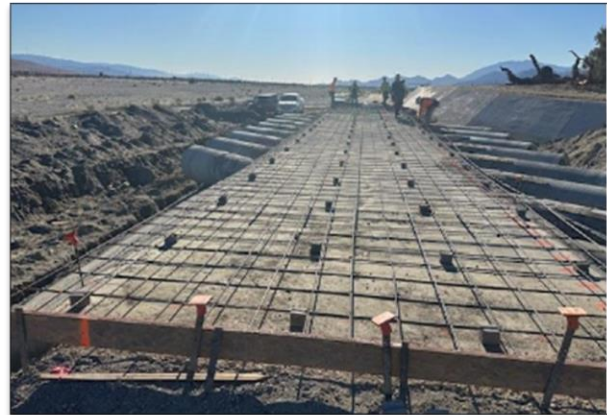
Setting rebar for structural concrete at in-channel crossing; Sunrise Way to Gene Autry.
