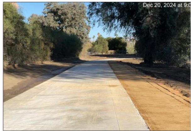
Grading 6' DG path on the dry side between west side of E Cielo and Mesquite in Palm Springs.
