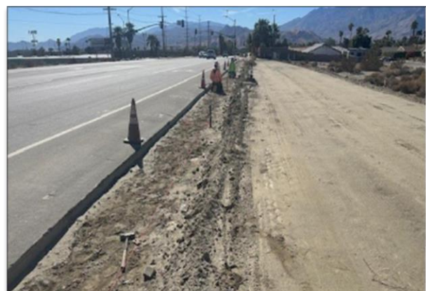
Setting forms for curb and gutter; North Palm Canyon to Indian Canyon.
