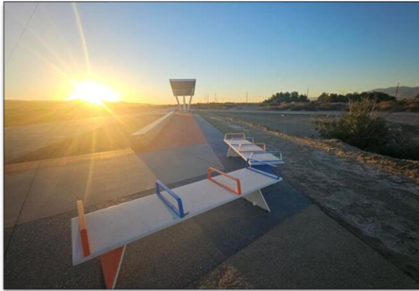
Install of shade structure, benches and bike rack at Ave 52 Access Point in Coachella.
