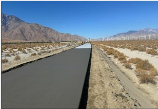
Placing Jointed Plain Concrete Paving; Indian Canyon to Gene Autry in Palm Springs.
