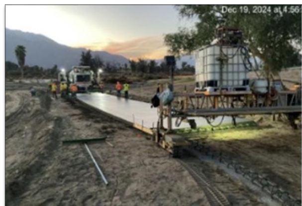
Placing Jointed Plain Concrete Paving 8" section on the west side of Cathedral Canyon.
