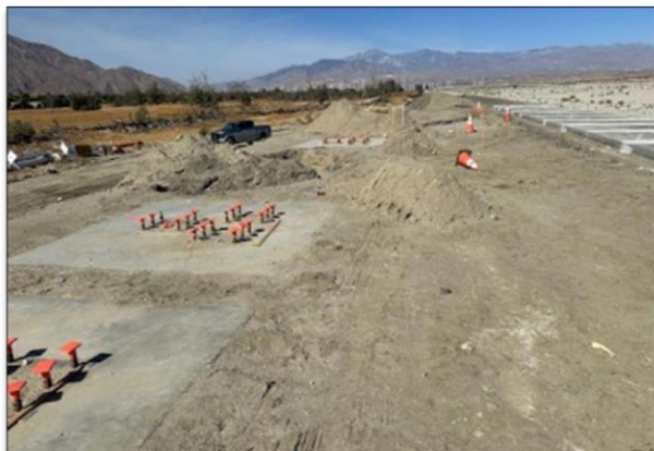
Grading and setting forms for minor concrete stadium seating structures; Whitewater Access Point.
