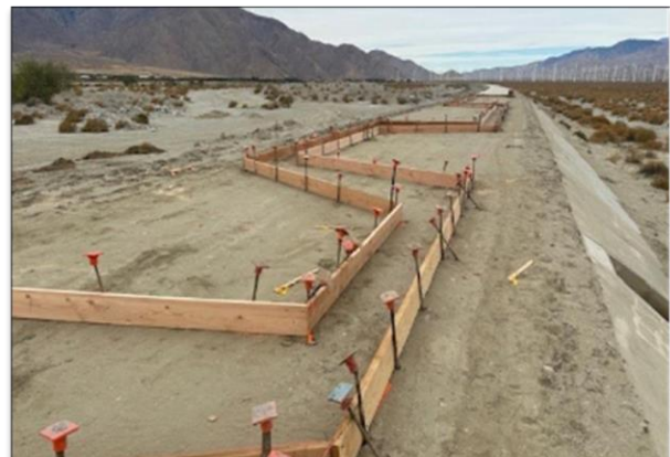
Laying out and installing forms for lithocrete; N. Palm Canyon to Indian Canyon.
