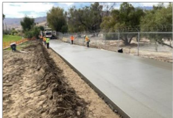
Placing Jointed Plain Concrete Paving on the West side of Lawrance Crossley
