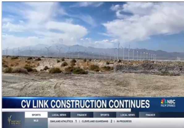
NBC Palm Springs coverage of CV Link construction start on segment 6 in North Palm Springs.
