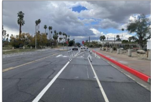
Delineators and striping upgrades added to the bike lane entrance of CV Link at El Cielo and Mesquite.
