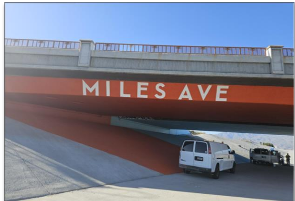
Miles Ave undercrossing painted in CV Link's signature orange and blue colors.
